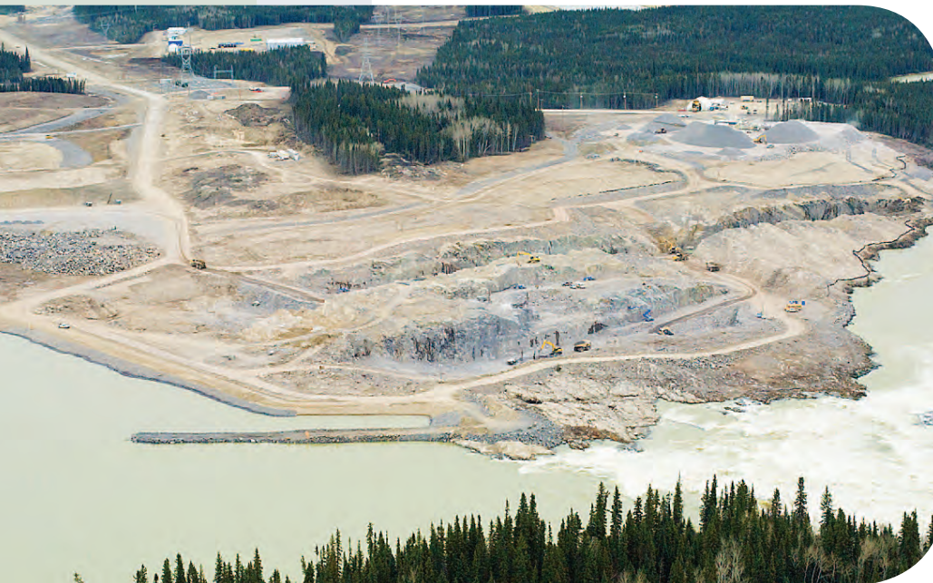
(top) The Wuskwatim Construction Camp, completed this year, is capable of housing over 700 project workers. Located adjacent to Wuskwatim Lake, it has many services and amenities.
