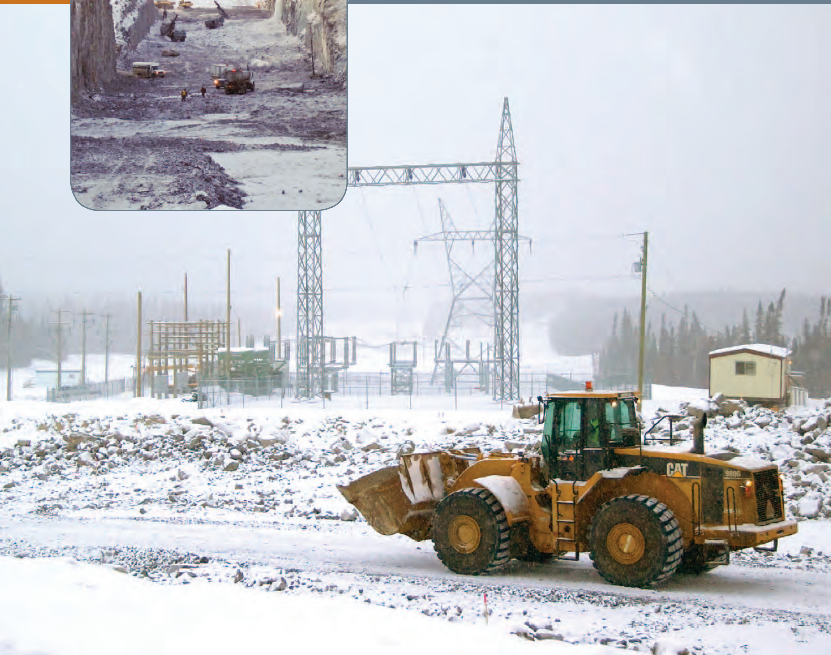
Northern Manitoba winters present harsh conditions for project workers, but some operations like clearing the right of way for transmission lines must be done in winter when the ground is frozen to prevent unnecessary disturbance.
