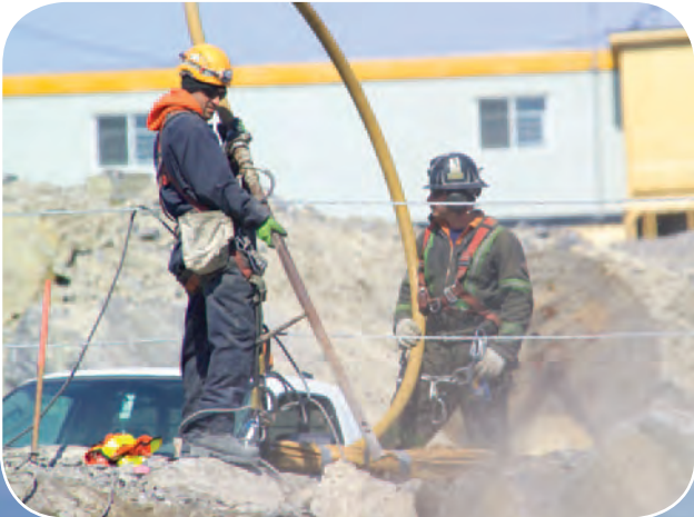
Workers using compressed air to remove loose rock and debris in excavation area.
