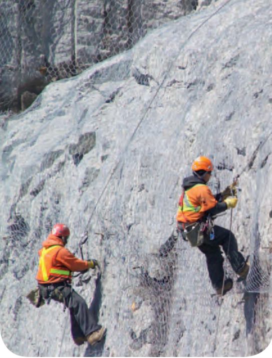
Construction workers suspended on rock face in spillway channel attach wire netting to secure loose rock.
